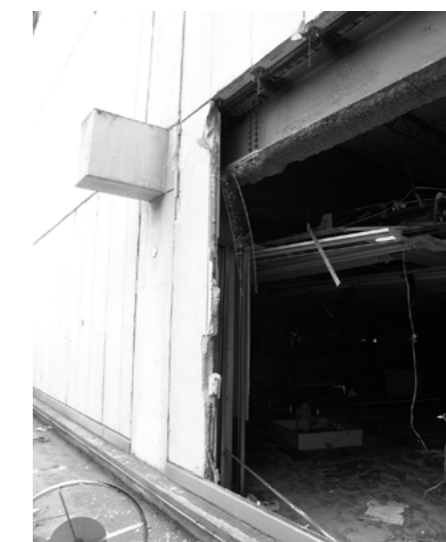
Figure 4. Damaged car park building for a commercial facility in Ofunato City, Iwate prefecture, caused by the Great East Japan Earthquake. Although the ALC panels suffered no damage from the earthquake, the tsunami broke through the wall and washed away the cars parked inside. This building was also of rebar-inserted longitudinal wall construction.
