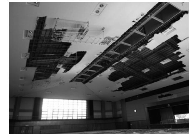
Figure 2. Ceiling collapse and damage at a gymnasium (the Great East Japan Earthquake, 2011) 1)
