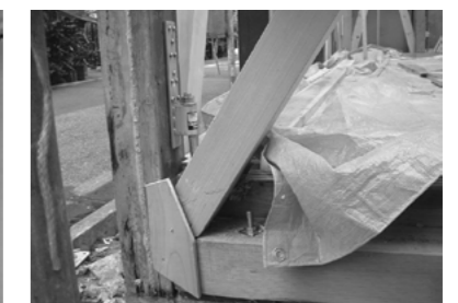
Figure 5. There are still many sub-standard seismic retrofit works.
