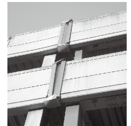
b) Deformation of a wall finishing panel of an EXP. J (photo: Tsuyoshi Seike)
