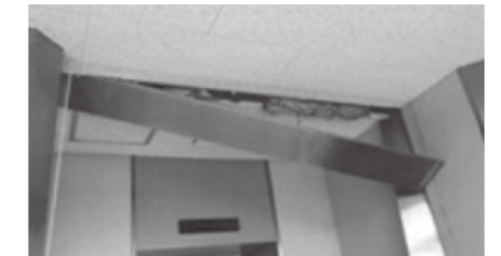
a) The ceiling finishing panel of an EXP. J has peeled off (photo: Satoru Ishiyama, Akita Prefectural University) 1)
