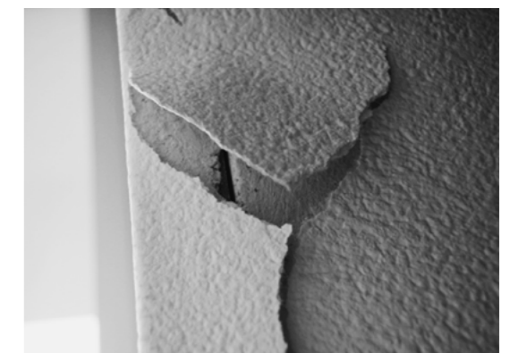
Figure 4. Partition walls with backings of light gauge steel in the hallway of super high-rise condominiums were broken.
