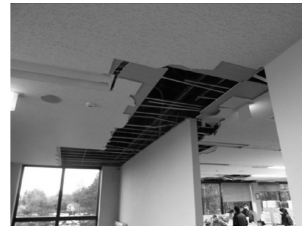
Figure 1. Damage to the ceiling at the top of a partition wall (the Great East Japan Earthquake, 2011) 1)
