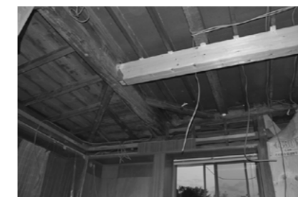
Figure 3. Lack of a beam on the second floor was found after the work started, and a beam was added.
