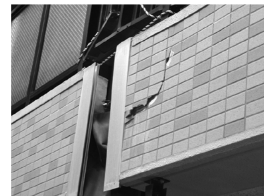
Figure 3. Balustrade wall at an expansion joint was broken.
