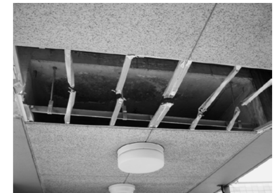
Figure 2. Ceiling materials at an expansion joint were broken and dropped off.
