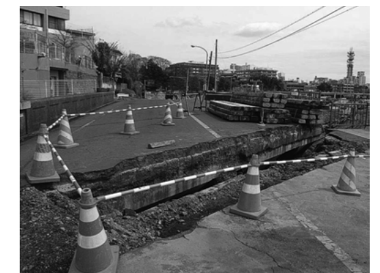
Figure 2. Difference of level caused by settlement of back filling under a bridge
