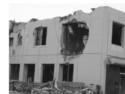
Figure 6. Exterior wall of relatively new reinforced concrete building which was destroyed by floating wreckage
