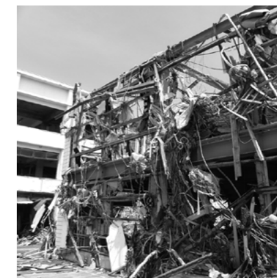
Figure 2. The exterior finish of the steel frame building was washed away, and wreckage was trapped by the structure.
