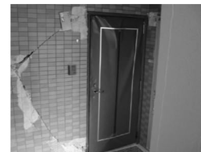
Figure 4. The entrance door has out-of-plane deformation, caused by cracked non-structural walls pushing on the door corners. The door can be forced open with a crowbar from outside, but it cannot be locked, leaving the premises insecure.
