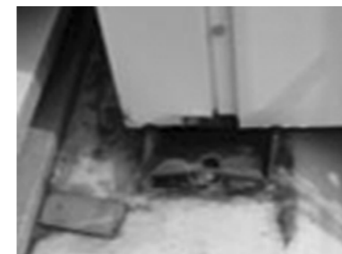
Figure 4. Fracture of base member of the equipment at the connection to the anchor bolts
