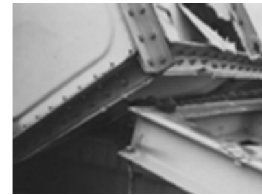
Figure 1. Anchor bolts came off
