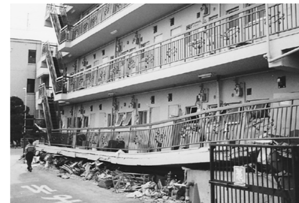
Figure 1. An example of the story collapse of the pilotis part of the ground story
