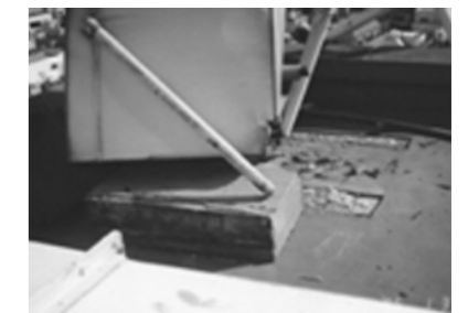
Figure 6. Overturning of beam-shape concrete foundation
