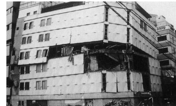
Figure 1. Collapse of PC CW
