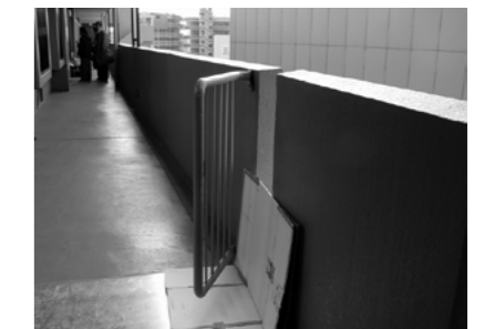
Figure 3. The expansion joint was damaged. The deformation of the balustrade shows signs of very severe shaking.
