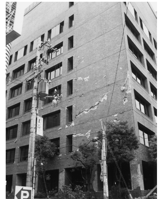
Figure 3. Damage to tile finishing which had been directly attached to the building frame
