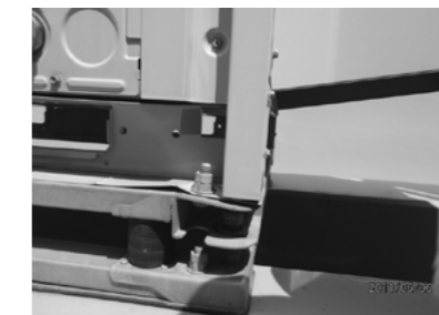
Figure 5. Deformation of vibration isolation base due to deformation of the equipment base member
