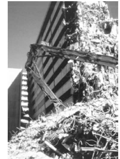
Figure 2. The speed of demolition after the Great Hanshin-Awaji Earthquake raised public suspicions.
