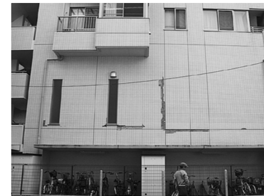
Figure 1. Tiles around earthquake-resistance slits were broken and dropped off.
