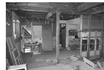
Figure 1. The state immediately after construction commenced. Construction started from the interior work leaving exterior walls as they were.
