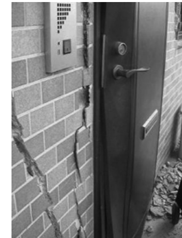
Figure 1. Damage to a front door (the Great East Japan Earthquake, 2011) 1)
