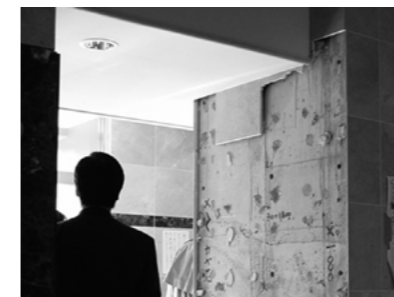
Figure 1. Wall finishes in the first story entrance hall fell off scattering rubble on the floor and blocking the designated evacuation route through the entrance hall.
