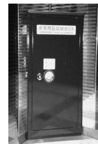
Figure 2. Storage box for emergency installed in an elevator. They were installed after the Great East Japan Earthquake as a countermeasure against being confined.
