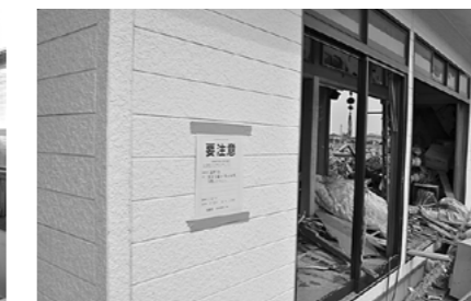
Figure 2. A house classified as "requires care" after tsunami damage
