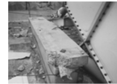
Figure 2. Damage of the corners of the concrete foundation
