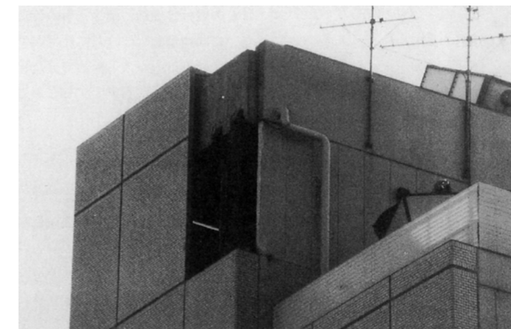
Figure 2. Falling of CW at a corner 1)
