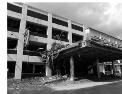
Figure 2. The City Hall of Rikuzentakata in Iwate prefecture suffered from flooding higher than the roof and was unable to function.
