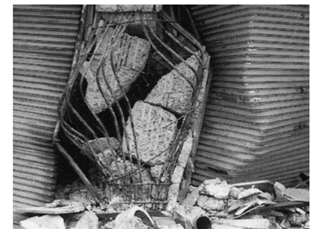
Figure 2. Hoops with spacing of 30 cm before 1970 (photo by: Faculty of Engineering, Tokyo Denki University) 1)
